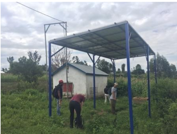
Figure 5.18: Municipal Tank & Pump
