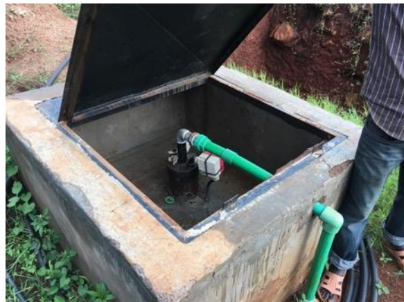
Figure 5.10: Private Electric Pump Installed by WECCO
