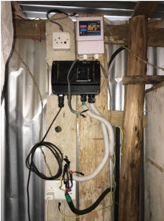
Figure 5.9: Electric Pump & Well
